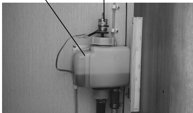
Expansion tank Circulation pump
